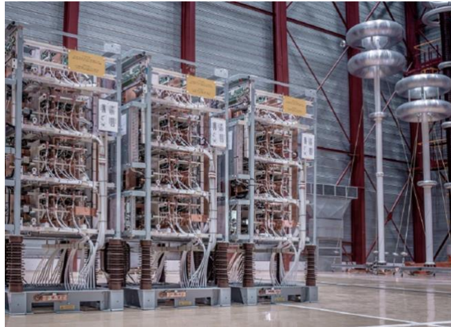
Figure 13 : MM7 converter towers from GE Power Conversion [7].
